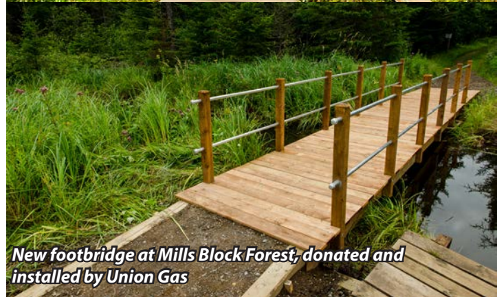
Union Gas Helping Hands In Action volunteers undertaking work at Mills Block Forest
