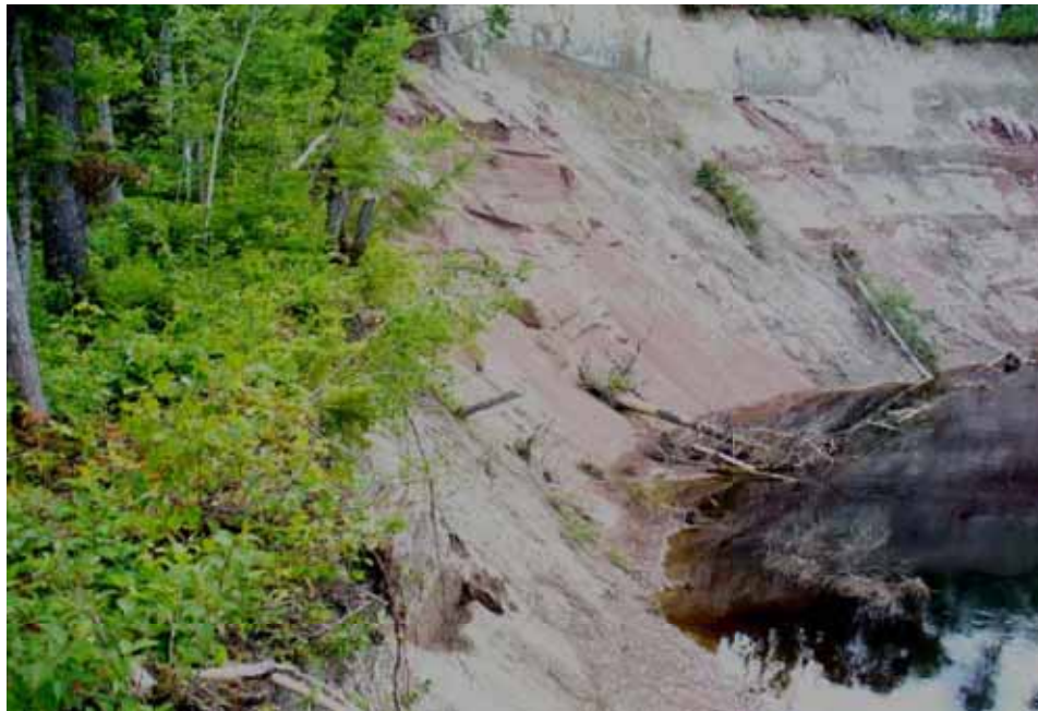
Figure 12: Bank Failure Prior to Remediation (LRCA 2008)
