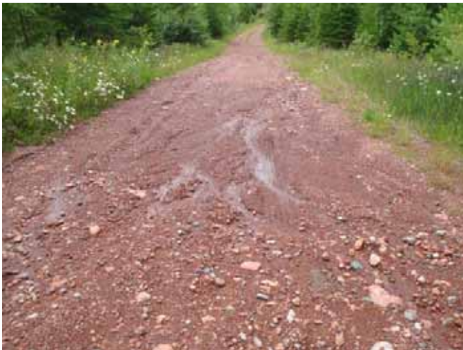
Site 6 Rills forming after rain on slope near sample Site 6.
