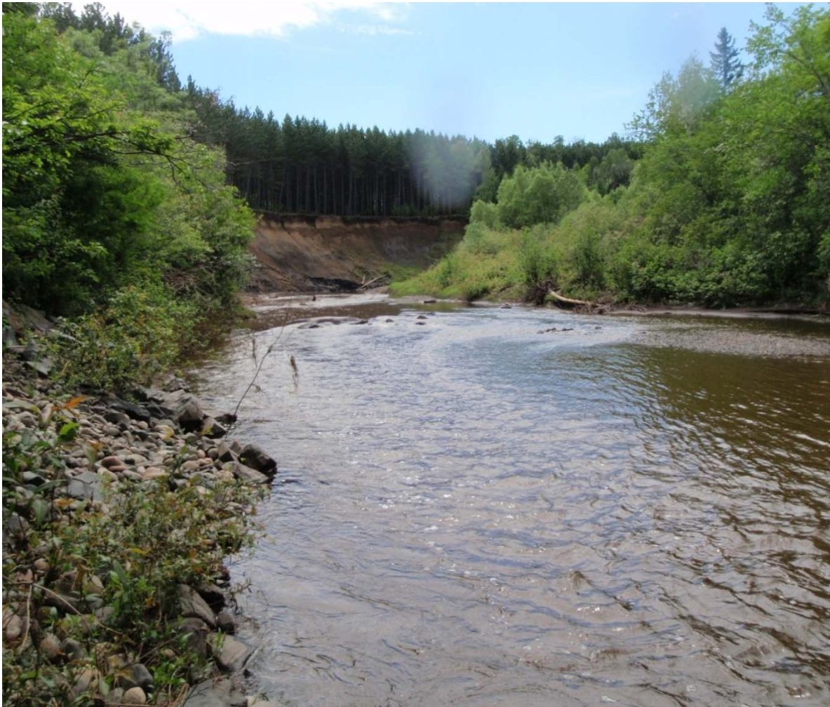
Figure 10: Bank Erosion Upstream at Site 6
