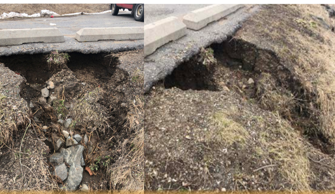
Examples of erosion (bank scour), at Mounddale Boat Launch.
