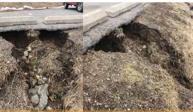
Examples of erosion (bank scour), at Mountdale Boat Launch.
