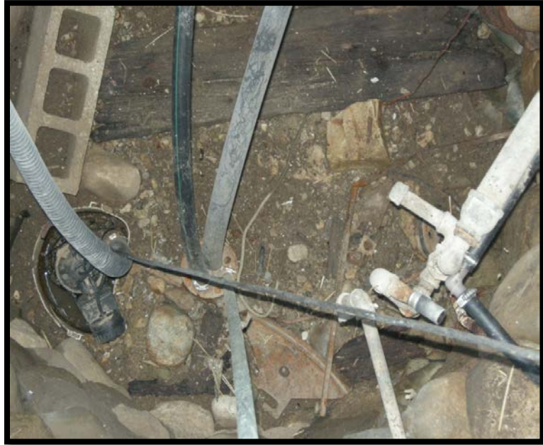
Poorly maintained wells can provide a conduit for contaminants to travel from the surface down to the aquifer. (SGSNBP Source Protection Region)
