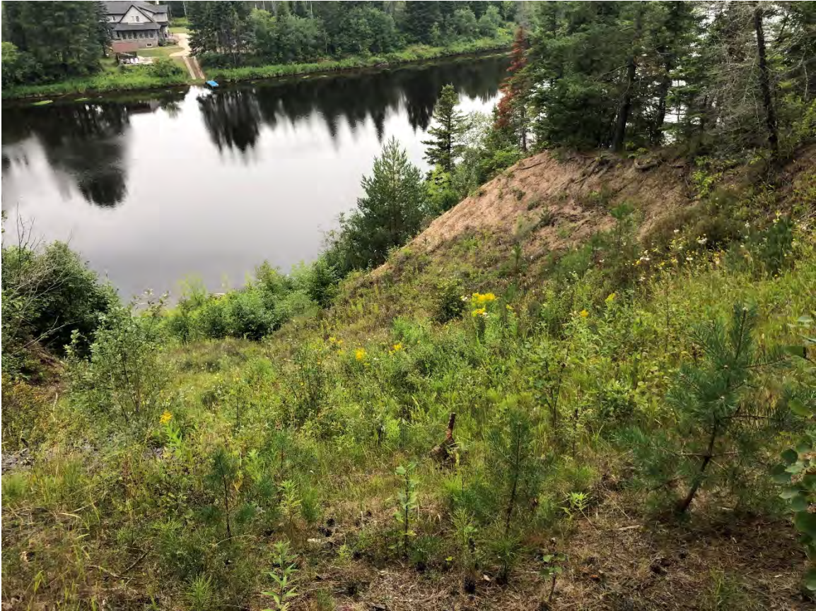
Site 2; add topsoil, fill and level. Keep existing young conifers and add vegetation to slope.
