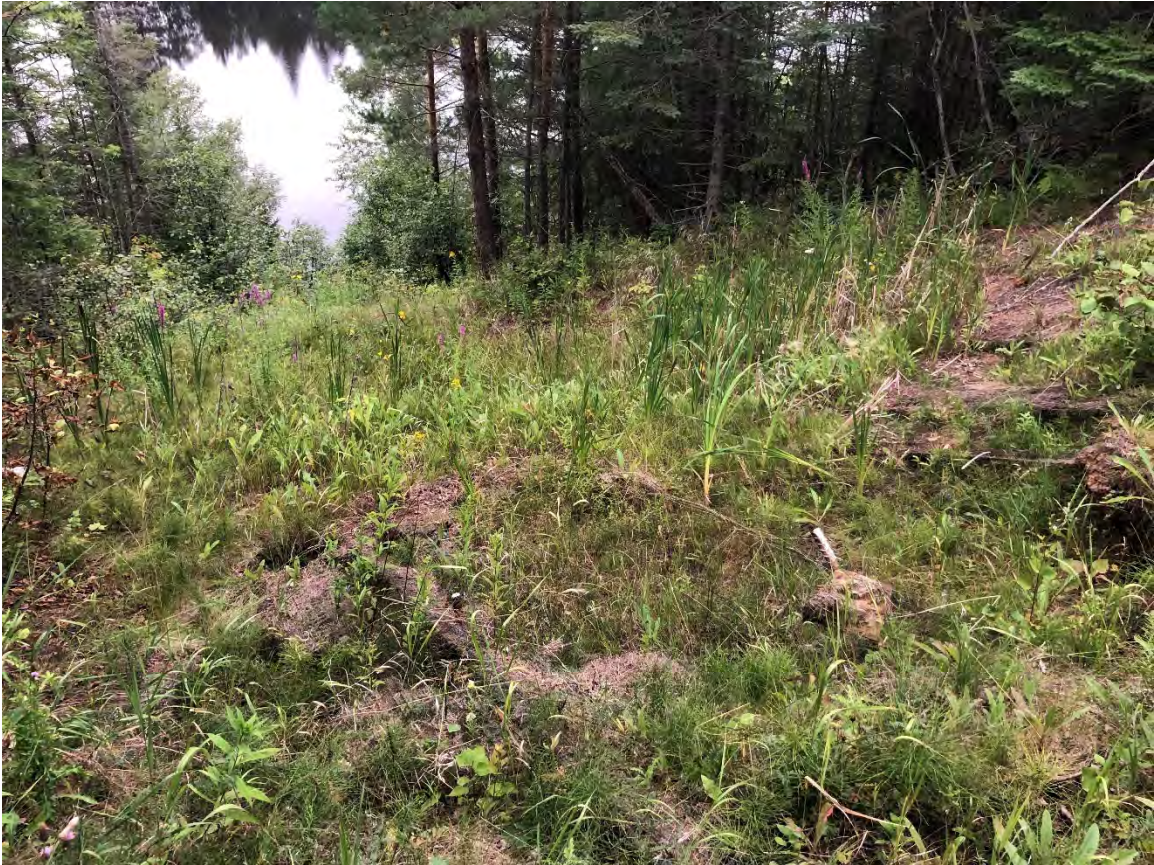
Site 1 where rip rap, geotextile, and adjustments to soil nail are needed.
