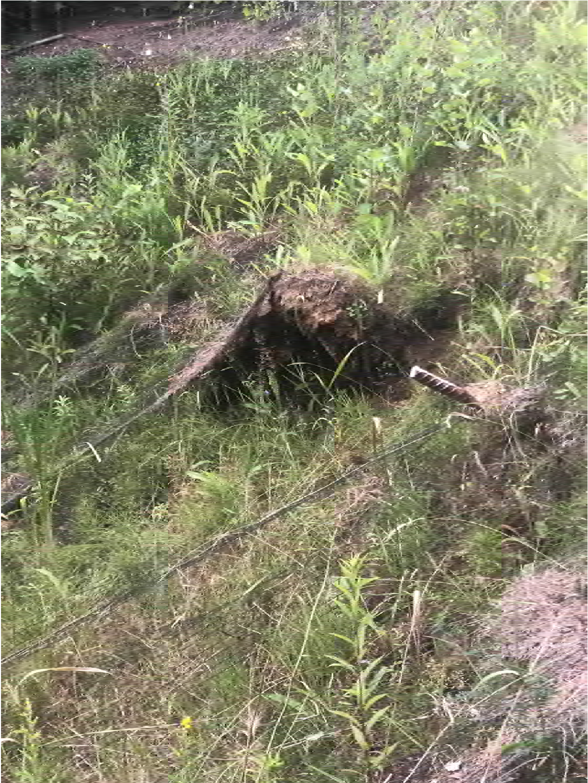
Soil nails and mesh requiring alterations at Site 1.
