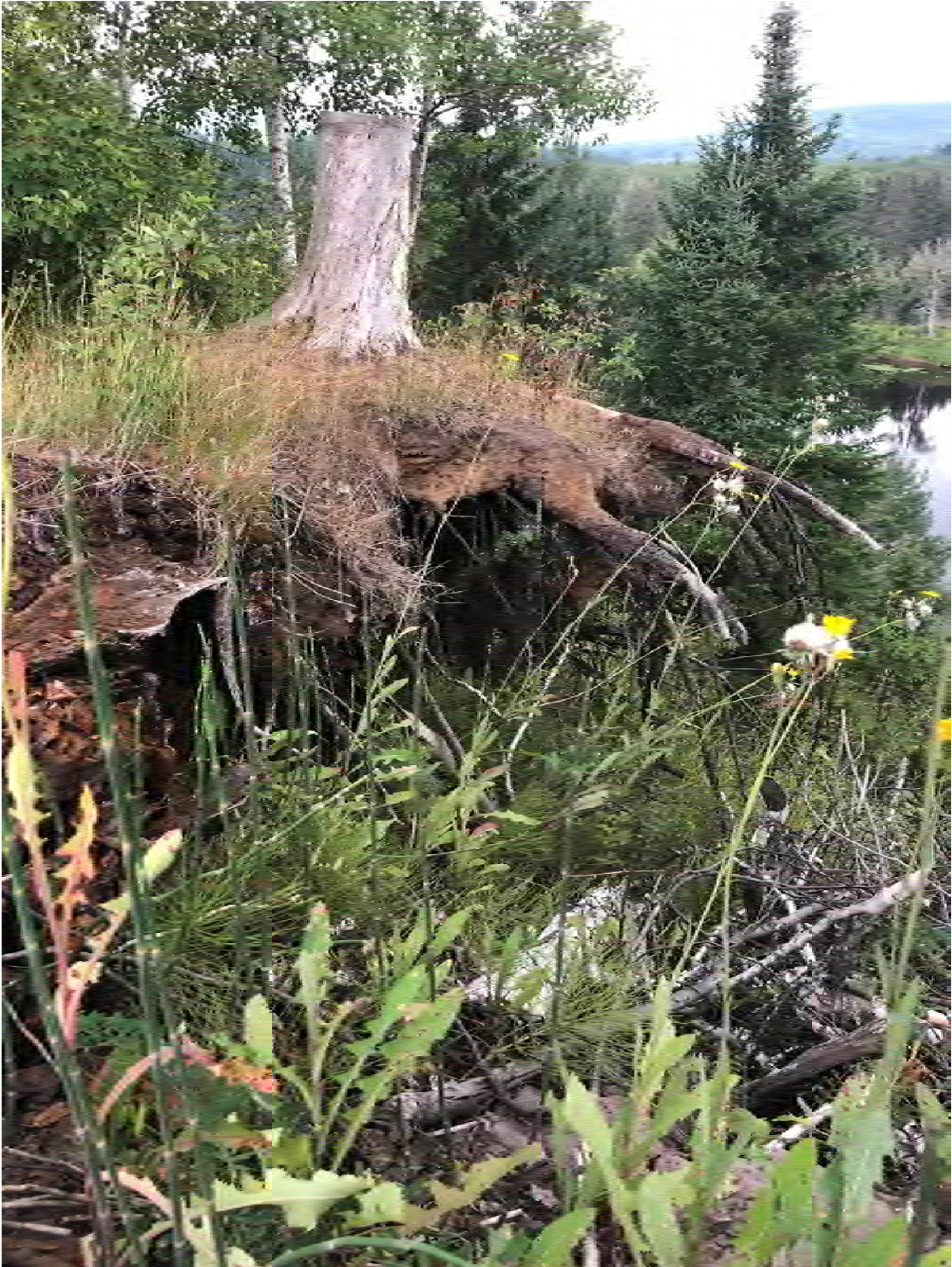
Erosion at 1610 Victor Street along Kaministiquia Riverbank.
