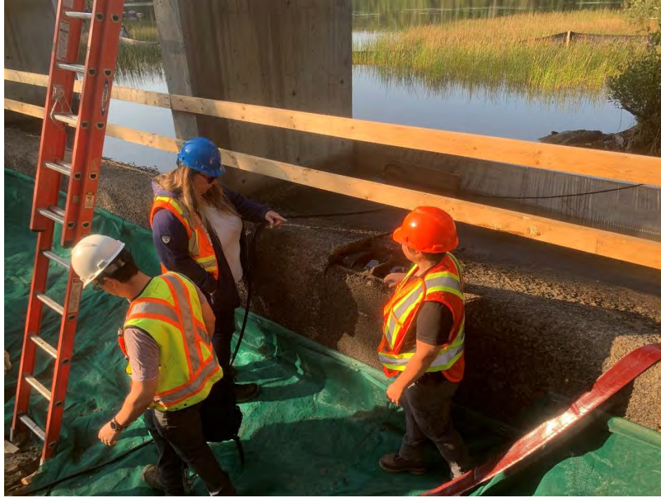
Photo 13: LRCA Staff conducting site visit at Hazelwood Dam with structural engineer from KGS
