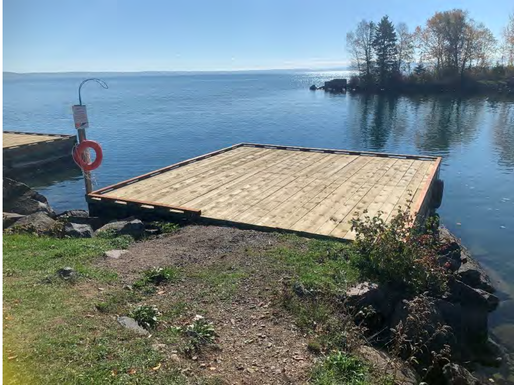
Photo 11: New Decking of Stationary Dock at Silver Harbour, one of three docks completed
